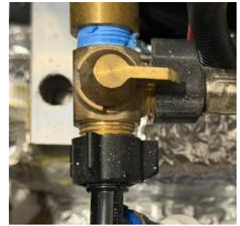
Water Heater Bypassed Winterization
