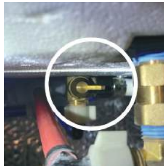
Water Heater Bypassed
