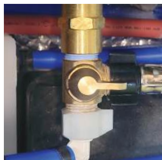
Water Heater Bypassed
