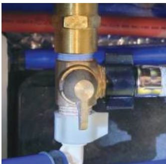
Valve Open (Allows water into water heater)
