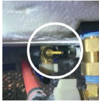
Water Heater Bypassed (Does not allow water into water heater)
