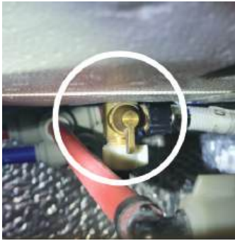
Valve Open (Allows water into water heater)
